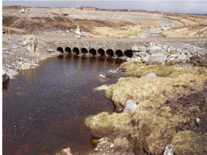
Figure 31 ✓ Good practice piped ford / causeway
