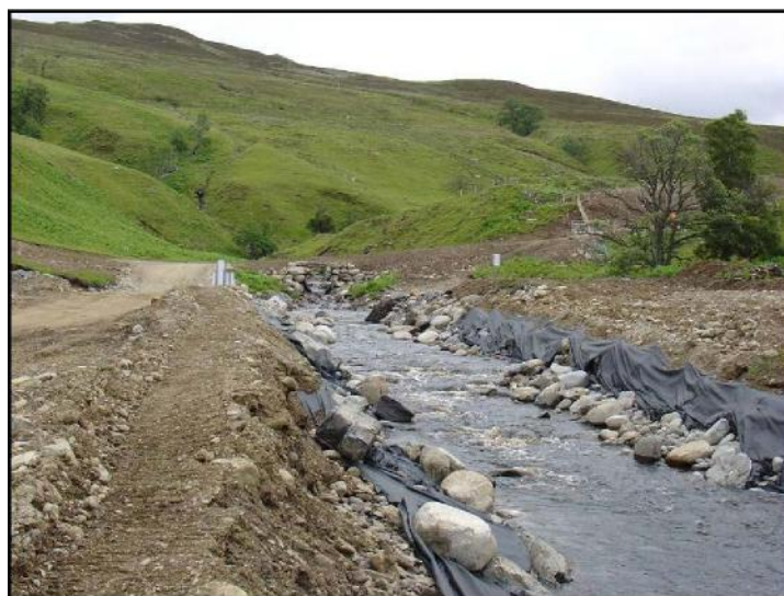
Figure 20 Full isolation by temporary diversion (NB The geotextile lining should extend to the full bank height and be properly secured.)
