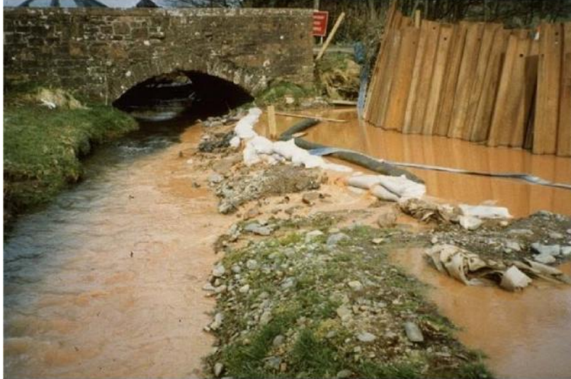
Figure 1 X Poor practice on a construction site leading to polluted surface water run-off
