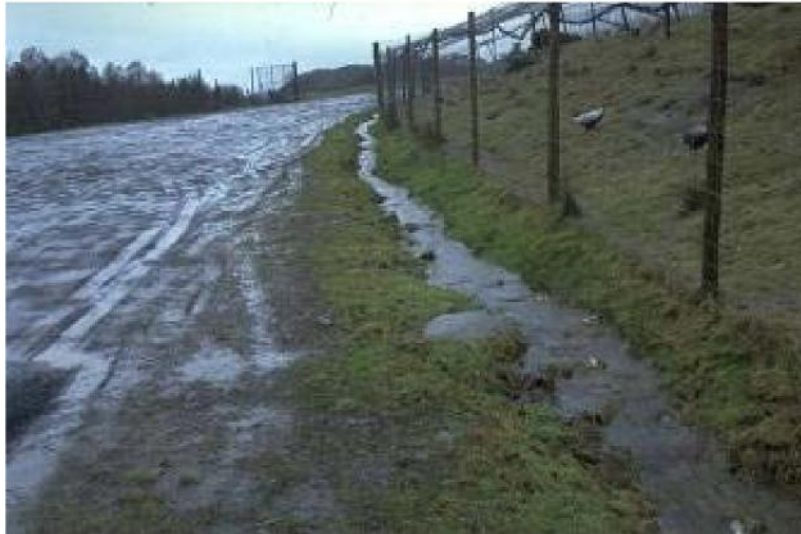
Figure 6 ✓ Good practice: diversion ditch along access road to intercept polluted water and carry to a treatment area
