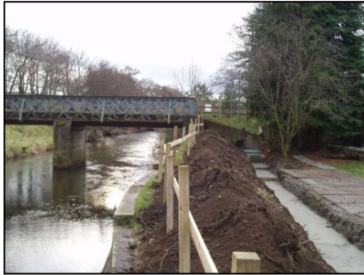
Figure 5 X Poor practice: topsoil from excavations stockpiled beside river leaving risk of pollution from run-off or high flow
