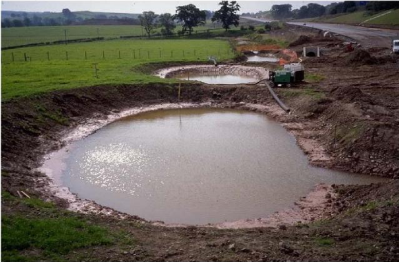
Figure 23 ✓ Good practice: series of settlement ponds
