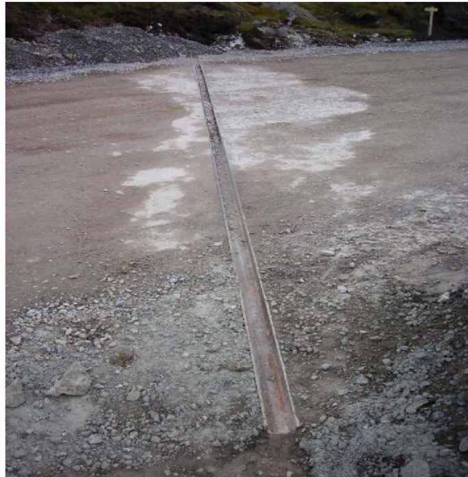
Figure 7 ✓ Good practice: cut-off drain on haul route to prevent erosion and direct polluted surface water to diversion drains or treatment areas (photo courtesy of Scottish and Southern Energy)
