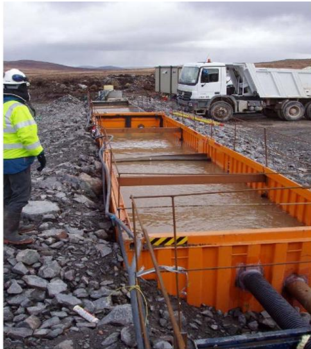
Figure 24 ✓ Good practice: settlement tanks (photo courtesy of Scottish and Southern Energy)
