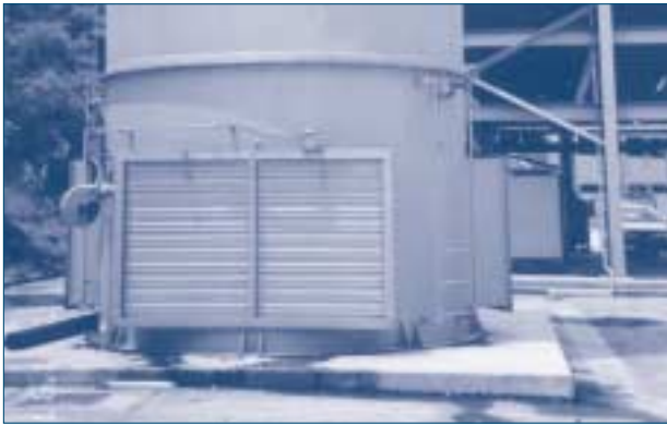
Figure 2.7 Automatically controlled combustion air louvres (often located inside the flare)
