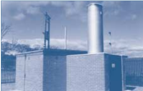
Figure A5.1 High-temperature, low-emissions enclosed flare within a brick enclosure to reduce noise impact
