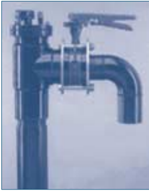
Figure 2.2 Typical landfill gas wellhead
