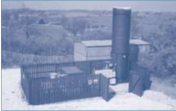
Figure 4.3 | Enclosed flare station
