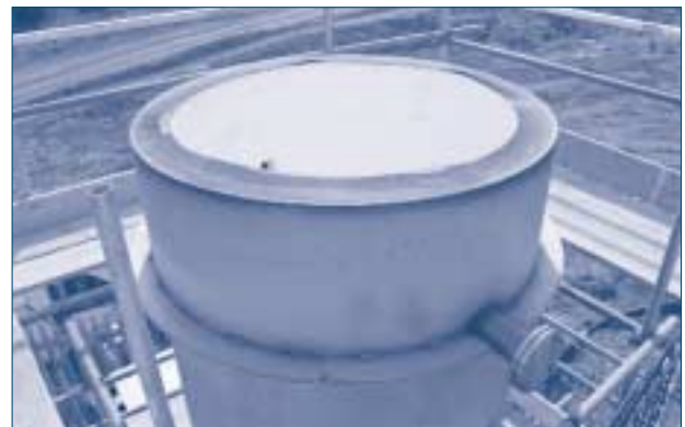
Figure 2.9 The top of an enclosed flare showing the refractory lining
