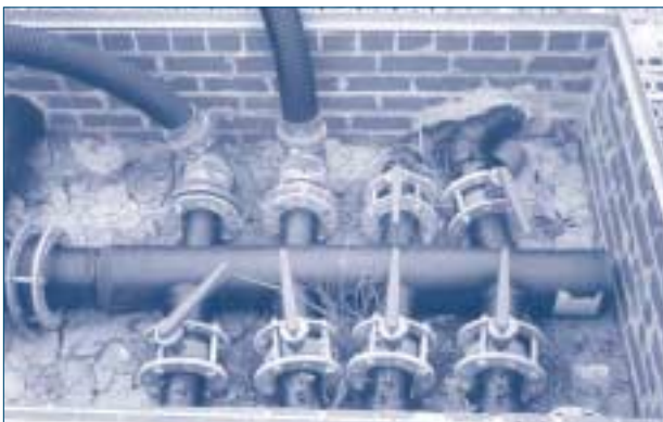
Figure 2.3 Typical landfill gas pipework manifold arrangement, used to control flow
