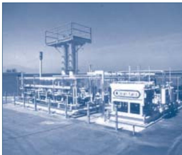
Figure 5.1 | Separex membrane separation plant at the Puente Hills landfill
