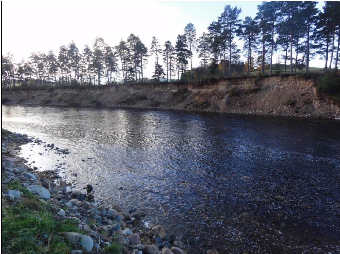
Figure 52: Severe erosion on the outside bend of the River Dee at Ballater immediately downstream from constriction caused by the embankment.
