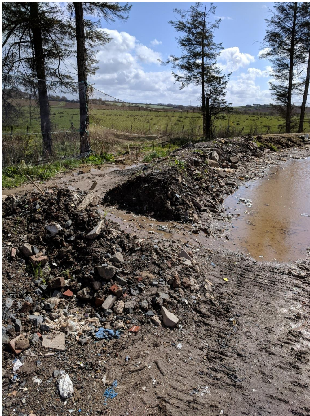
Figure 14 - Water logging along the east-south east site track, breached bund and water discharge off site
