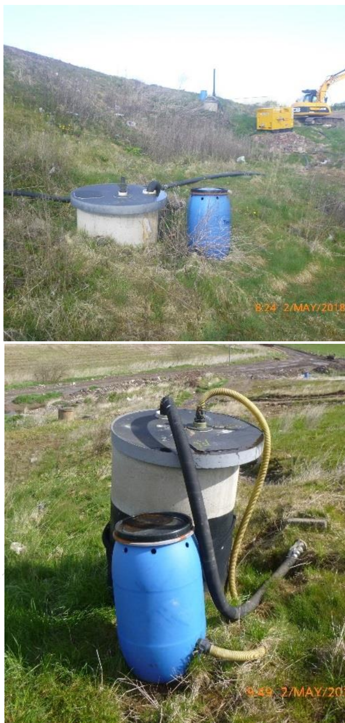
Figure 9 - Leachate wells LW15 (top) and LW12 (bottom) at Tarbolton Landfill site.
