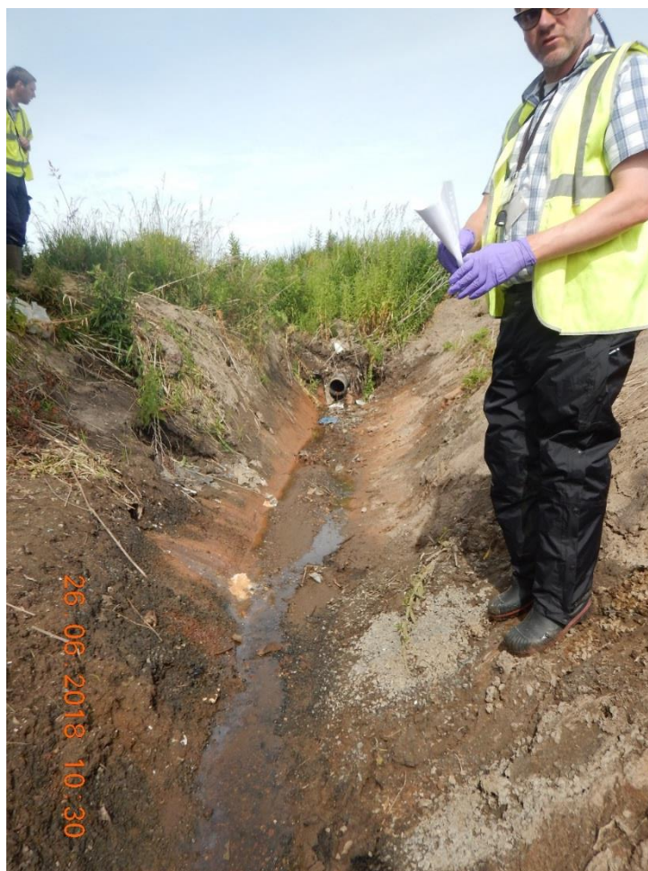
Figure B9 Photograph of surface water ditch showing one of the discharge pipes
