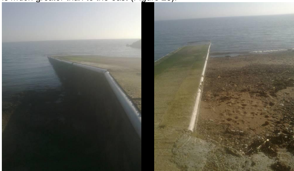
Figure 23: Western slipway showing different accumulation of sediment to the west.
