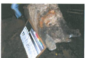
Spoil in Bucket Note Rust Color (42)
