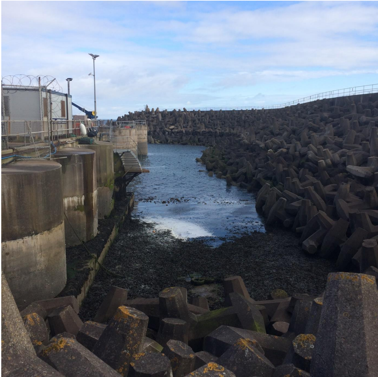
Figure A8vii Spume at the western side of the spillway (May 2016).
