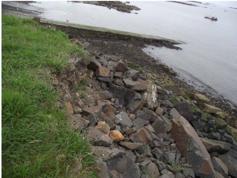
Figure 5 Promontory 1 Erosion (Chainage 170m) with Jetty beyond
