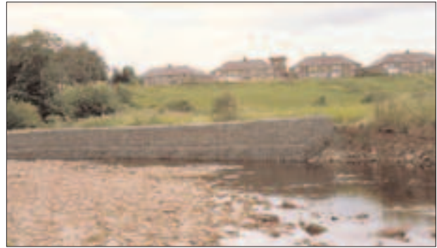
Figure 11 Erosion displaced to the end of a structure
