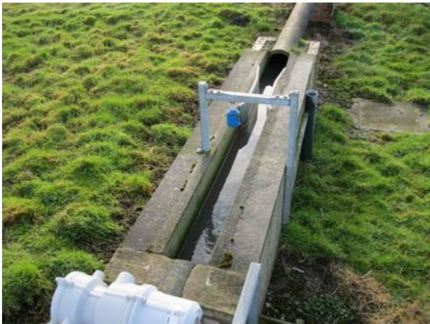
Figure 19 Rectangular Flume with upstream ultrasonic sensor
