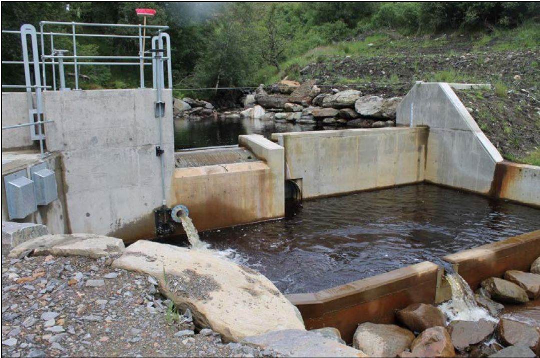
Photograph 1: Example intake and mitigation structure, showing the release of compensation flows via a pipe with orifice plate straight from the intake chamber.
