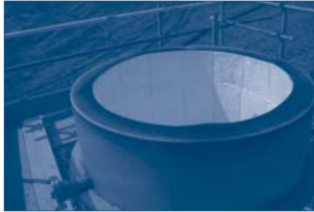
Figure 5.6 Top of flare shroud with sampling port with access platform in place
