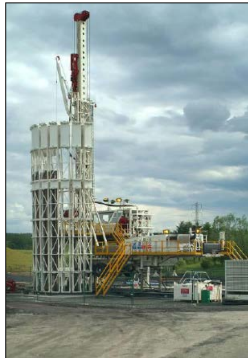
Figure 3- Drill rig used to construct deep boreholes in operation (From Dart Energy information)
