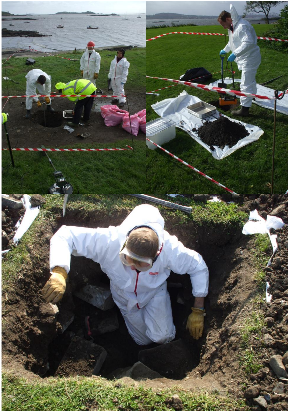
Figure 4. Site Excavation: Combined, digging and auguring (image top left); surface excavation (image top right); buried slabs of concrete (lower image).
