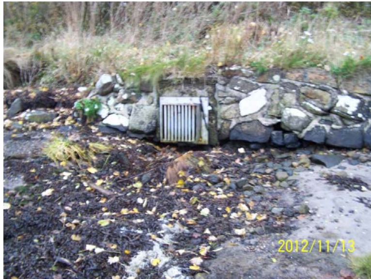
Figure 11 Spinneys SPS Emergency Outfall (Chainage 740m) – showing scour under wall
