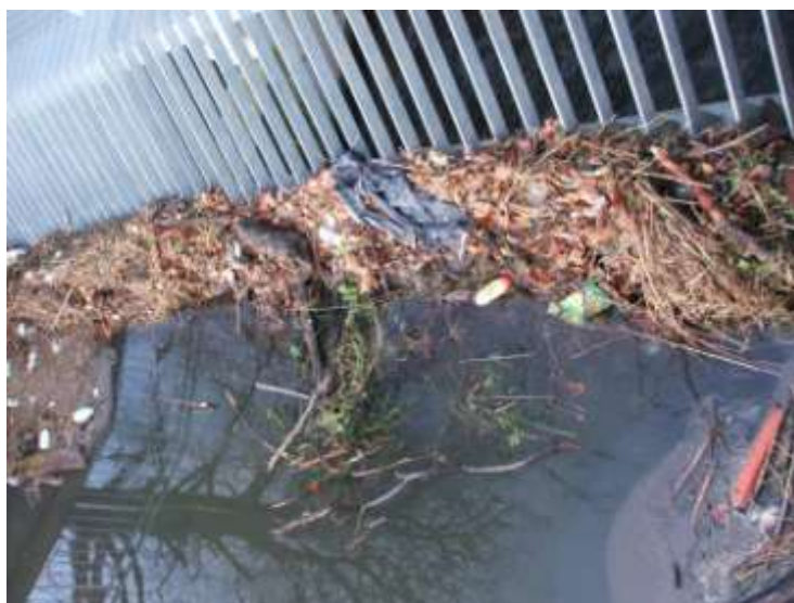
Figure 1-33: Trash on the screens on the culvert under the Old Dalkeith Road
