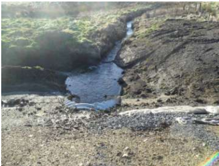
Figure 1-15: Morphological instability at the new road crossing of the Boghead Burn
