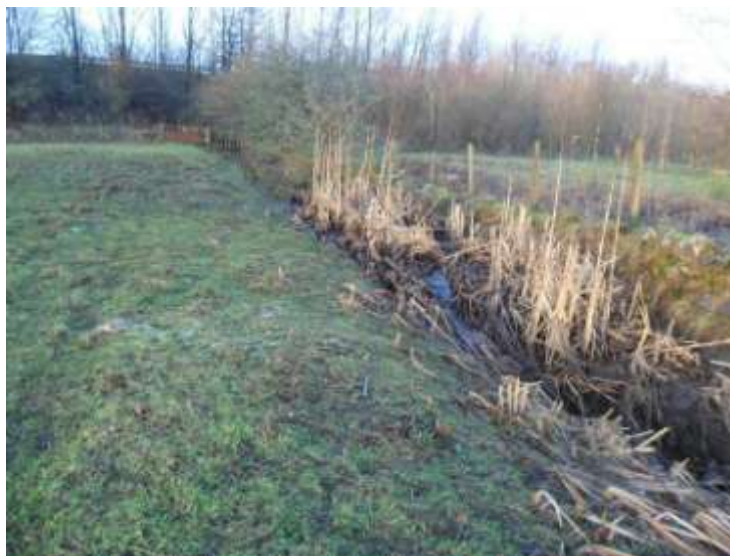
Figure 1-8: Reed covered in-channel sediment downstream of the A801 culvert
